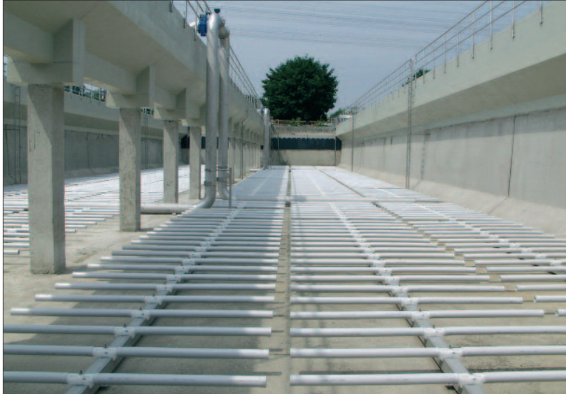
HANAU WASTE WATER TREATMENT PLANT: AERATED WITH MAGNUM®2000 FLEXSIL® MEMBRANE DIFFUSERS.
